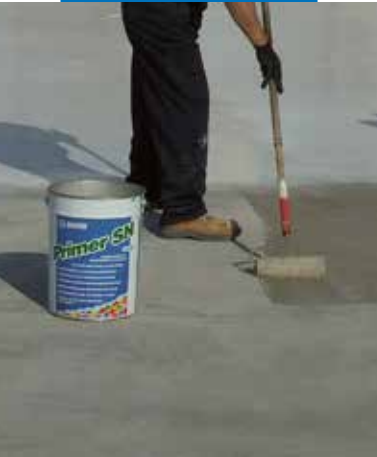
Application of Primer SN on a concrete floor slab with a roller
