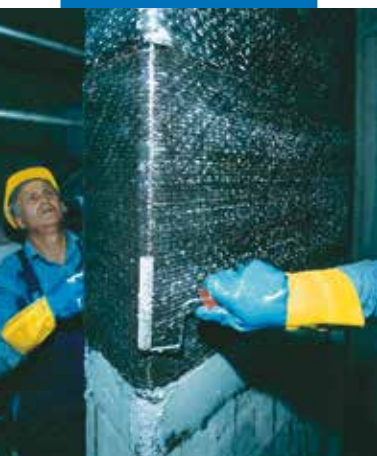
Applying pressure on the fabric with the Roller for MapeWrap so that MapeWrap 31 can penetrate well into the fabric
