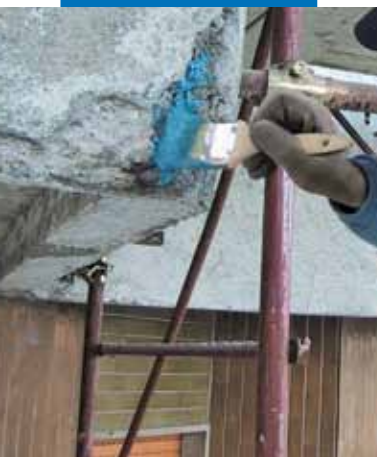
Applying Mapefer 1K with a brush on reinforcing rods on a reinforced concrete balcony
