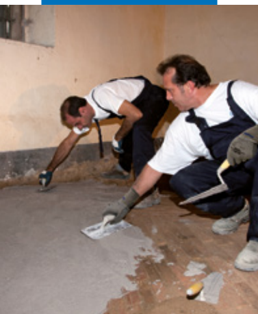
Application of the first layer of Planitop HDM Restauro by trowel on the outer face of a vaulted ceiling
