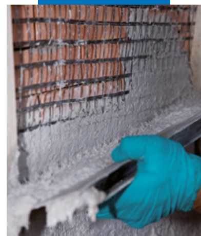
Application of Planitop HDM Restauro system with Mapegrid G 220 on a brick wall
